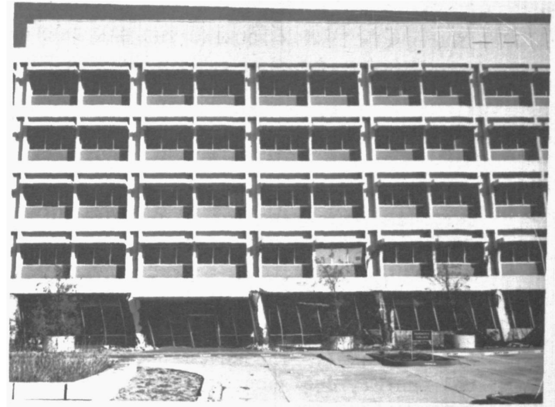
Olive View Hospital (First story has a permanent displacement of 2 feet (61 cm))
