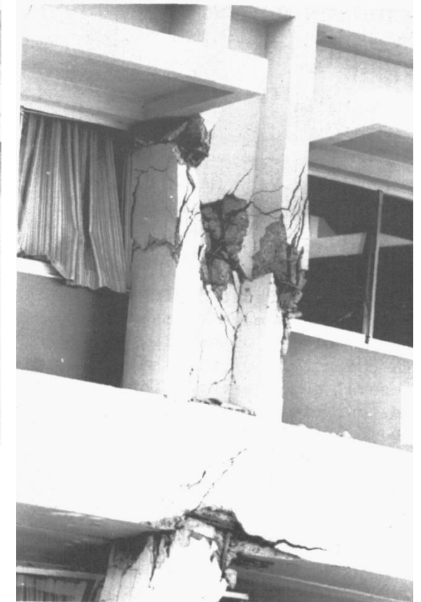
Second story column fracture in Olive View Hospital
