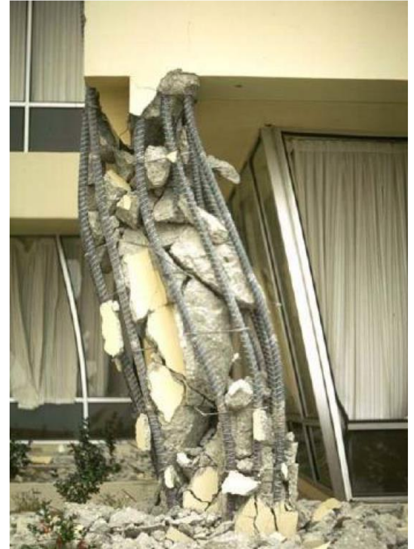
Column with inadequate ties Source: FEMA 451
