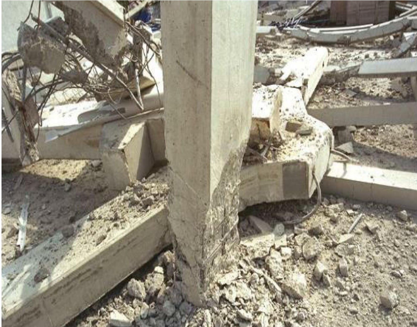
Severe spalling of column cover concrete exposing longitudinal steel. Source: FEMA P-58/BD-3.8.6
