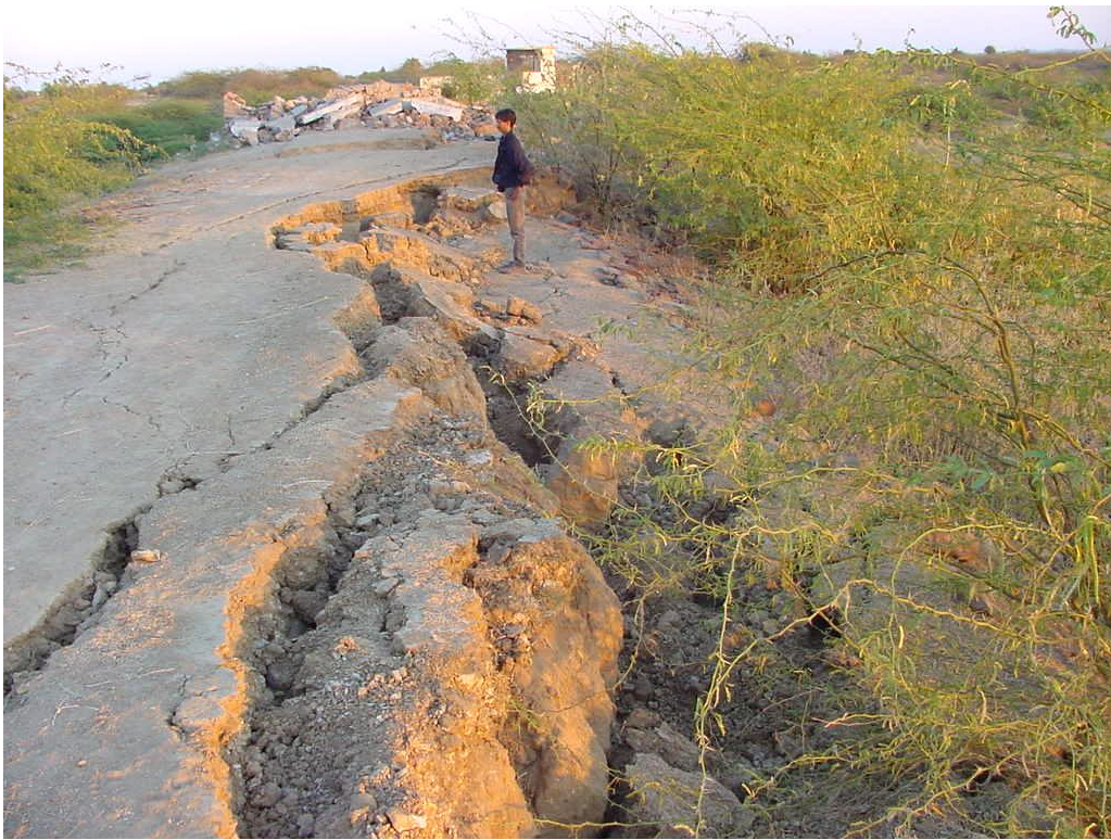
Bhuj earthquake 2001 Irrigation Dams
