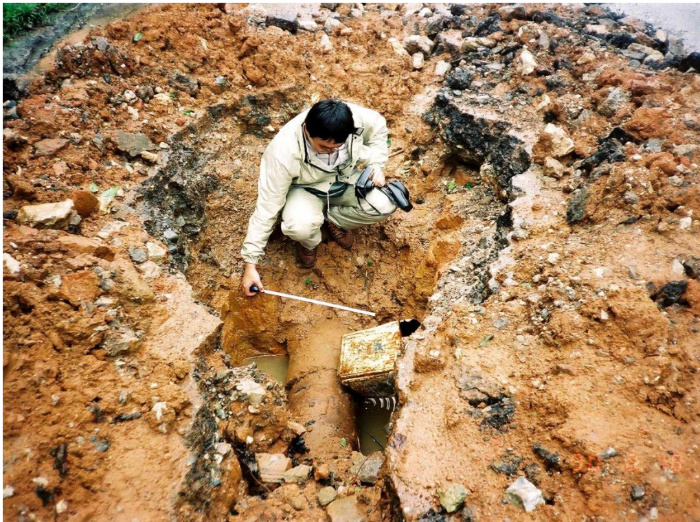
Underground Pipe Failure in Baguio, Philippines ( Luzon Earthquake, 1990 )
