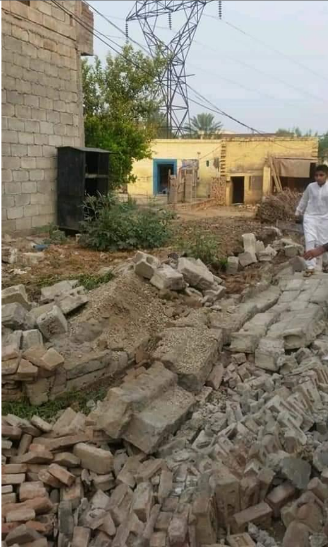
Collapse of block/brick masonry
