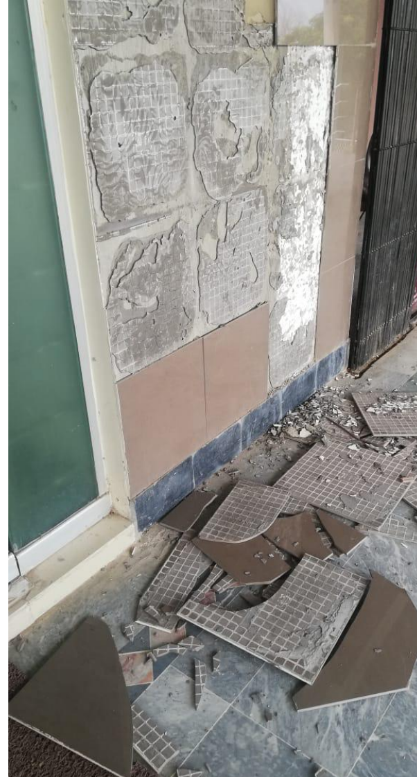
Spalling of tiles
